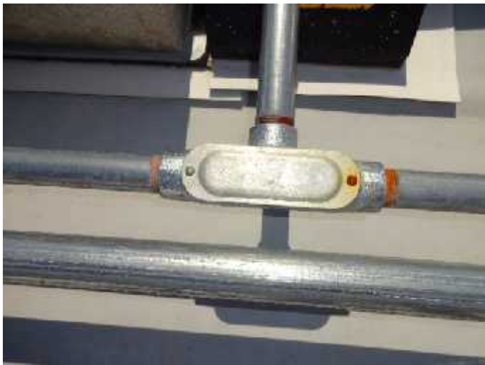
Exhibit 3. Visible Corrosion of Conduits and Hardware
